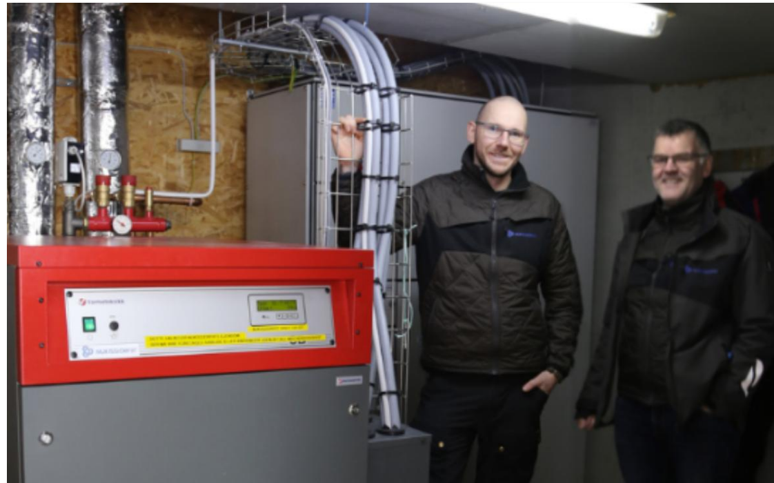
Figure 8: Deployment of an electric boiler at Hotel SØMA in Nuuk, replacing fuel oil and reducing CO 2 emissions by 142 tonnes annually (Nukissiofiit, 2024b)
